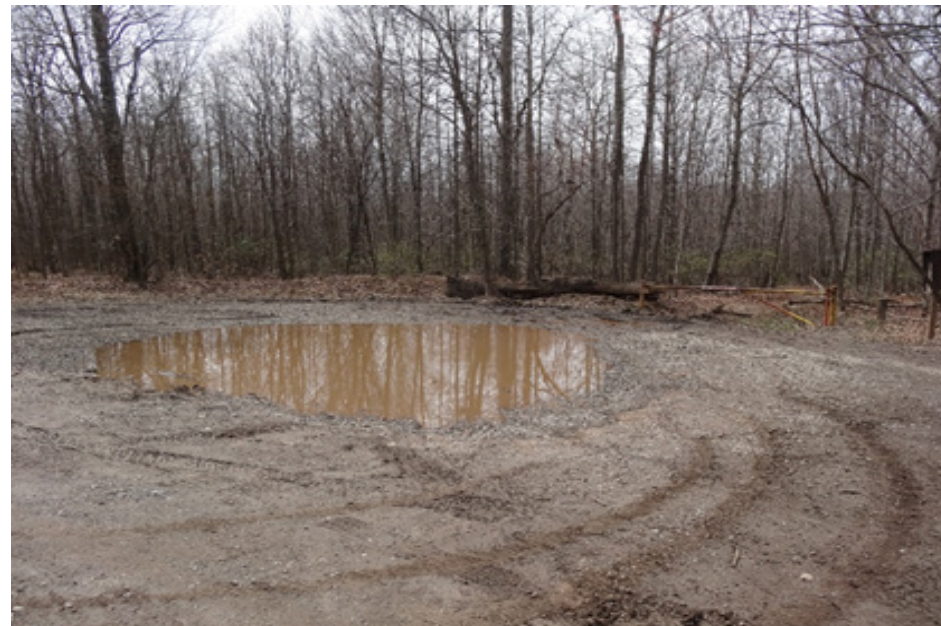
Figure 1. Overused, flooded guest-created parking
