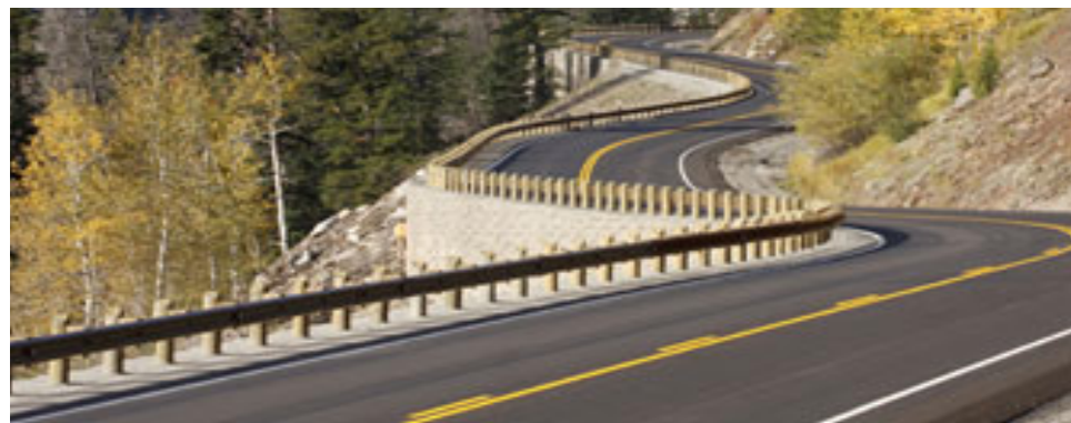
Figure 46: Rail Protection for safety.
