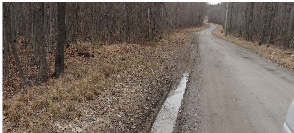
Figure 3. Road side erosion
