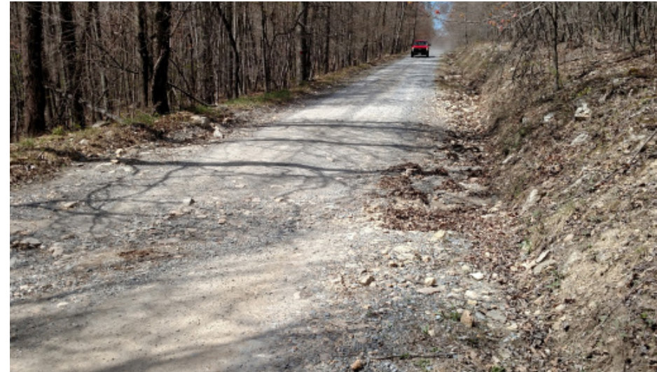
Figure 40: Deterioration of roadway due to steep slope.
